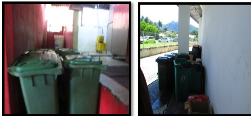
PICTURE 1. Limited waste storage space and inadequate bins
