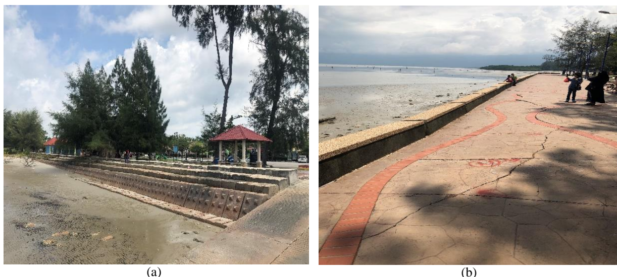
Figure 2. Current condition showing: (a) concrete block built as wave protection structure at Pantai Batu Laut; and (b) Sea walls showing signs of failure in Pantai Morib
